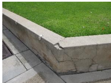
Retaining wall needs repairs
