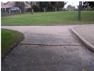
Walkways need repairs
