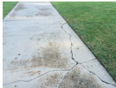
Pedestrian Paving needs repairs
