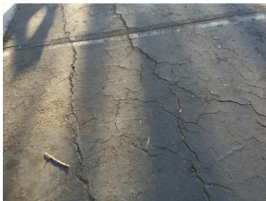
Asphalt needs repairs
