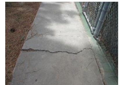
Pedestrian paving needs repair
