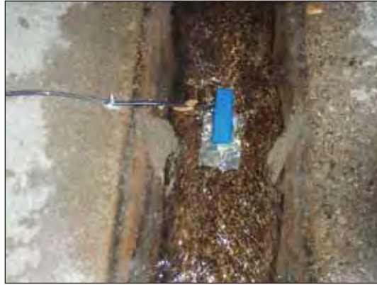
Figure B-3. Example of Sensor Installation
