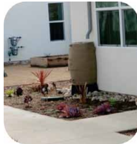
Figure 4-2 Rain Barrel Capturing Runoff From a Residential Property
